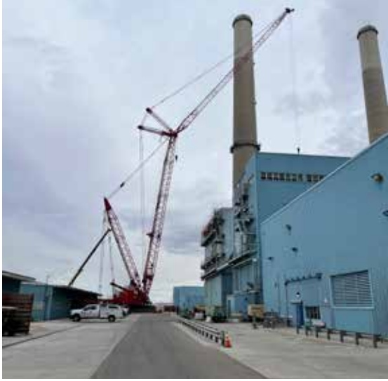
A crane set up at Laramie River Station to help with the overhaul of the plant's electrostatic precipitator.
