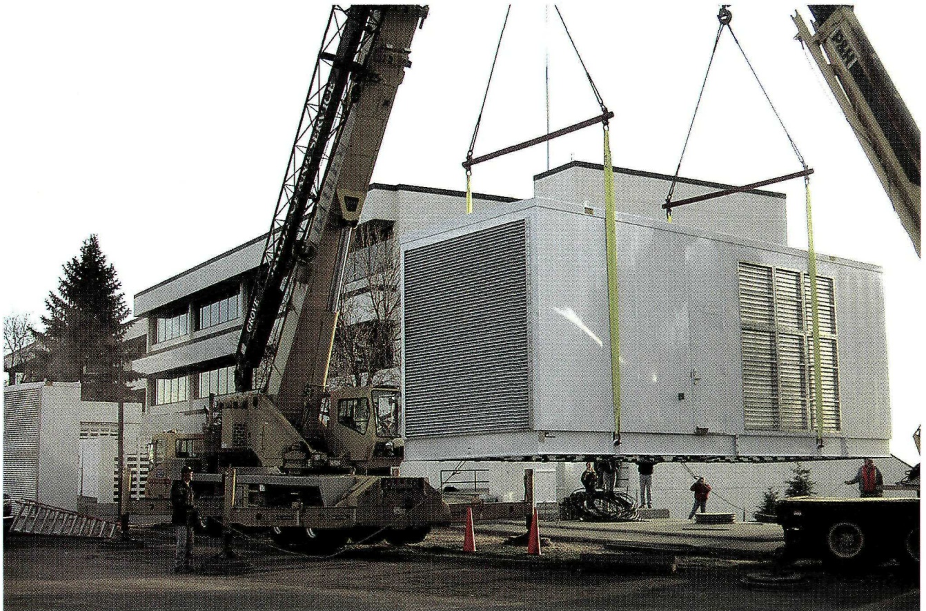
Two cranes move Basin Electric's new standby generator to a concrete pad adjacent to Headquarters. The 1500-kilowatt diesel-powered Caterpillar generator was installed Oct. 21. Leland Olds Station Unit 3, a mobile generator, powered Headquarters two weekends before and during installation. Capital Electric and Basin Electric crews were on hand to replace the majority of Capital Electric's power cabling surrounding Headquarters. A Capital Electric transformer, originally located near Headquarters' cooling tower, was moved near the receiving area to facilitate the installation .
