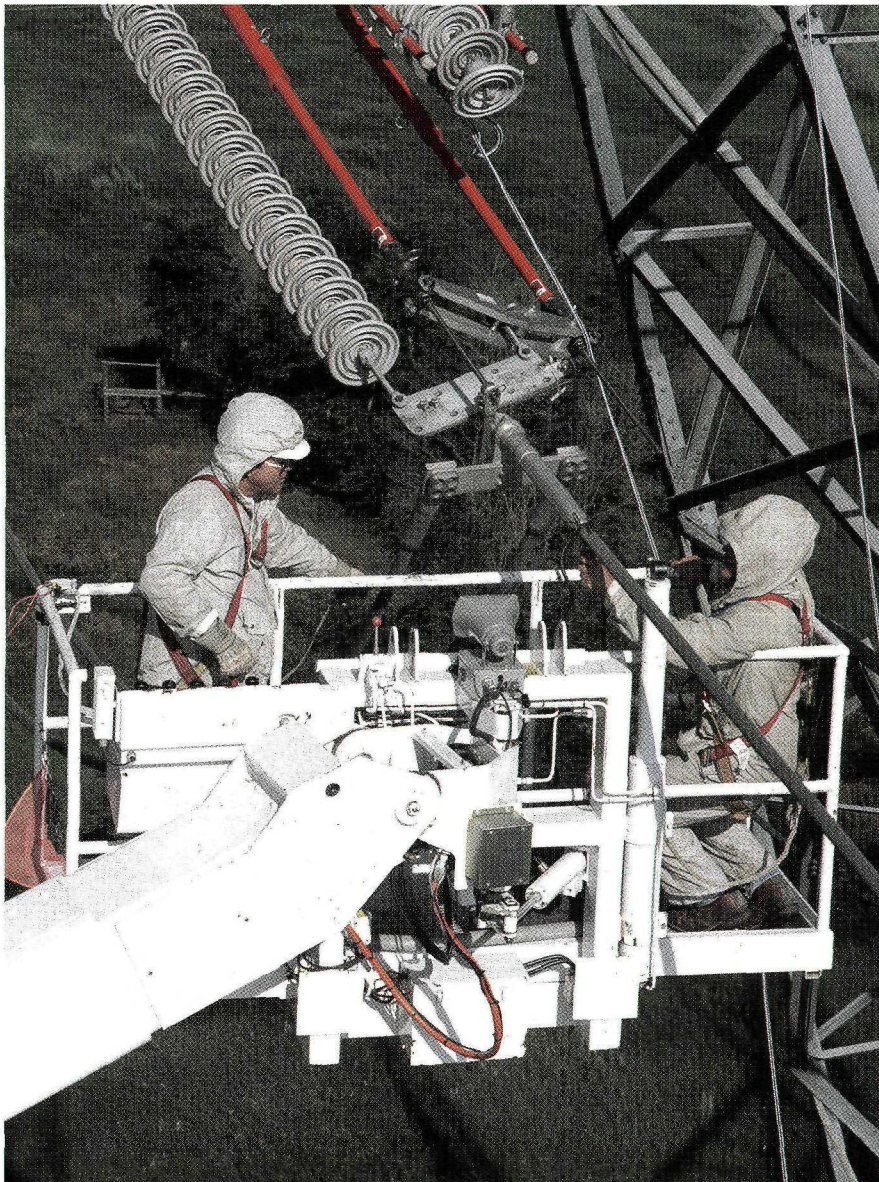
TSM employees change out an insulator on the Antelope Valley Station/Broadland 500-kilovolt (kV) line using the barehand and hotstick methods. The line is energized to 345-kV.
